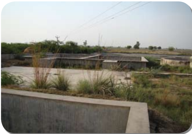
Pic 25: Water works (diggi) at village Sardana (Sonapat). Defunct since 1987, but is often repaired. 16.6.10
