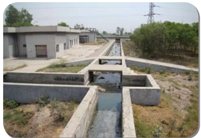
Pic 14: Idle 35 MLD STP at Panipat. 29.4.10
