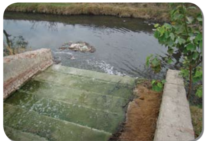
Pic 16: Treated effluent from 30 MLD STP at Sonapat is falling into the polluted waters of Drain no 6. (16.6.10)
